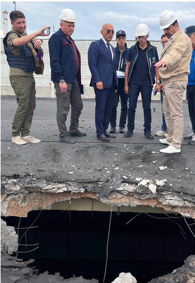
BELOW: IAEA team observes damage caused by shelling on the roof of the special building at the ZNPP that houses the fresh nuclear fuel and the solid radioactive waste storage facility. Credit: IAEA
