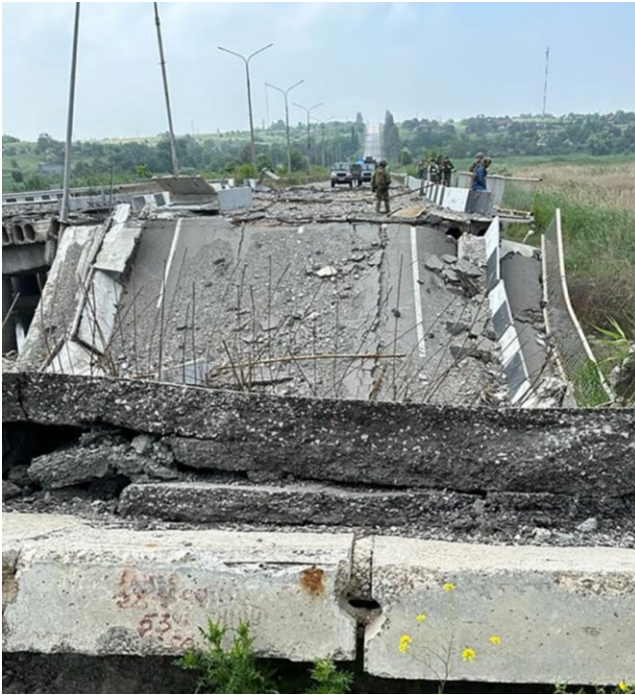
ABOVE: A broken bridge from shelling and air attacks near the Zaporizhzhya Nuclear Power Plant. 15 June 2023. Credit: IAEA
